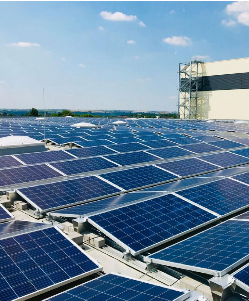
By using solar energy – as illustrated with solar panels at the location in Kitzingen – Schaeffler makes an important contribution to climate protection.
